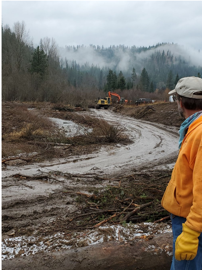
Photo 16: Construction. Streambank access road, left bank. Upstream of landowner property, facing upstream. (11.24.2020.jpg1.jpg)
