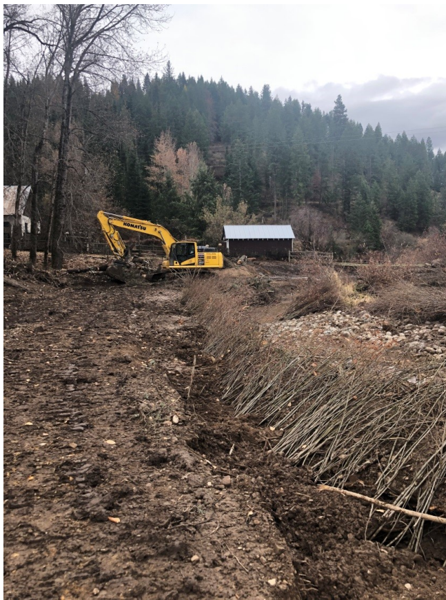
Photo 13: Construction. Recontouring of stream with Vegetated Wood Matrix Type 1 installation. Left bank, upstream of property owner, facing downstream. ( DownstreamMurphy.jpg )
