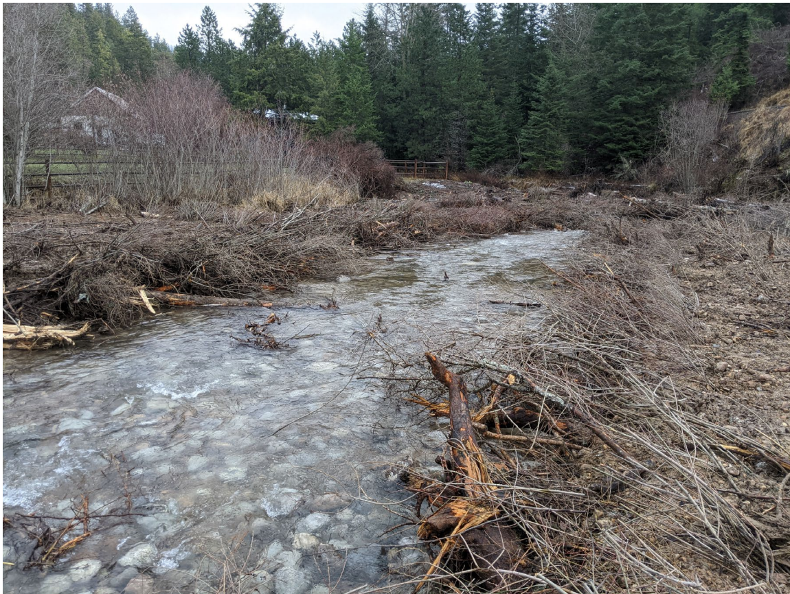
Photo 22: Post Construction. Installed Vegetated Wood Matrixes and constructed streambed downstream of property owner's structures. Facing downstream ( PXL_20201125_173543929.jpg )
