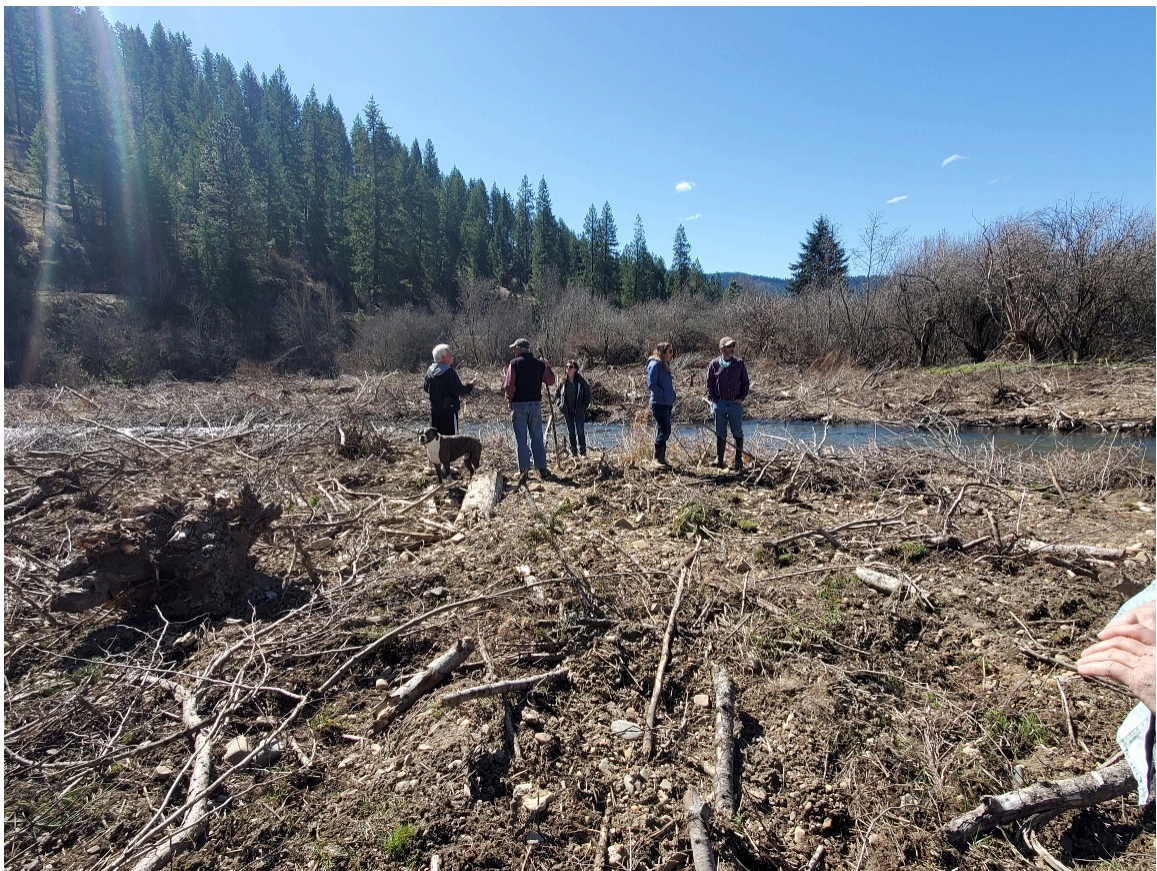
Photo 26: Post Construction Spring. Inspection with partners of left bank downstream of landowner's structures. ( Groupshot.jpg )
