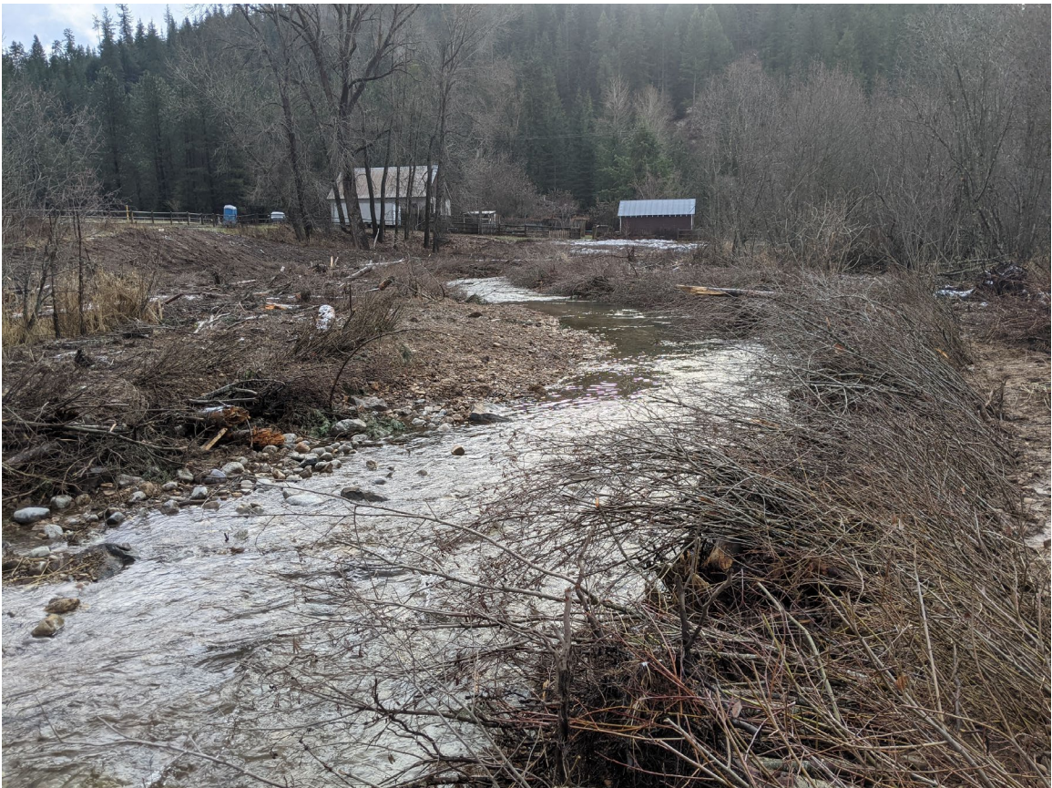
Photo 21: Post Construction. Installed Vegetated Wood Matrixes and constructed streambed upstream of property owner's structures. Facing downstream. ( PXL_20201125_172445806.jpg )
