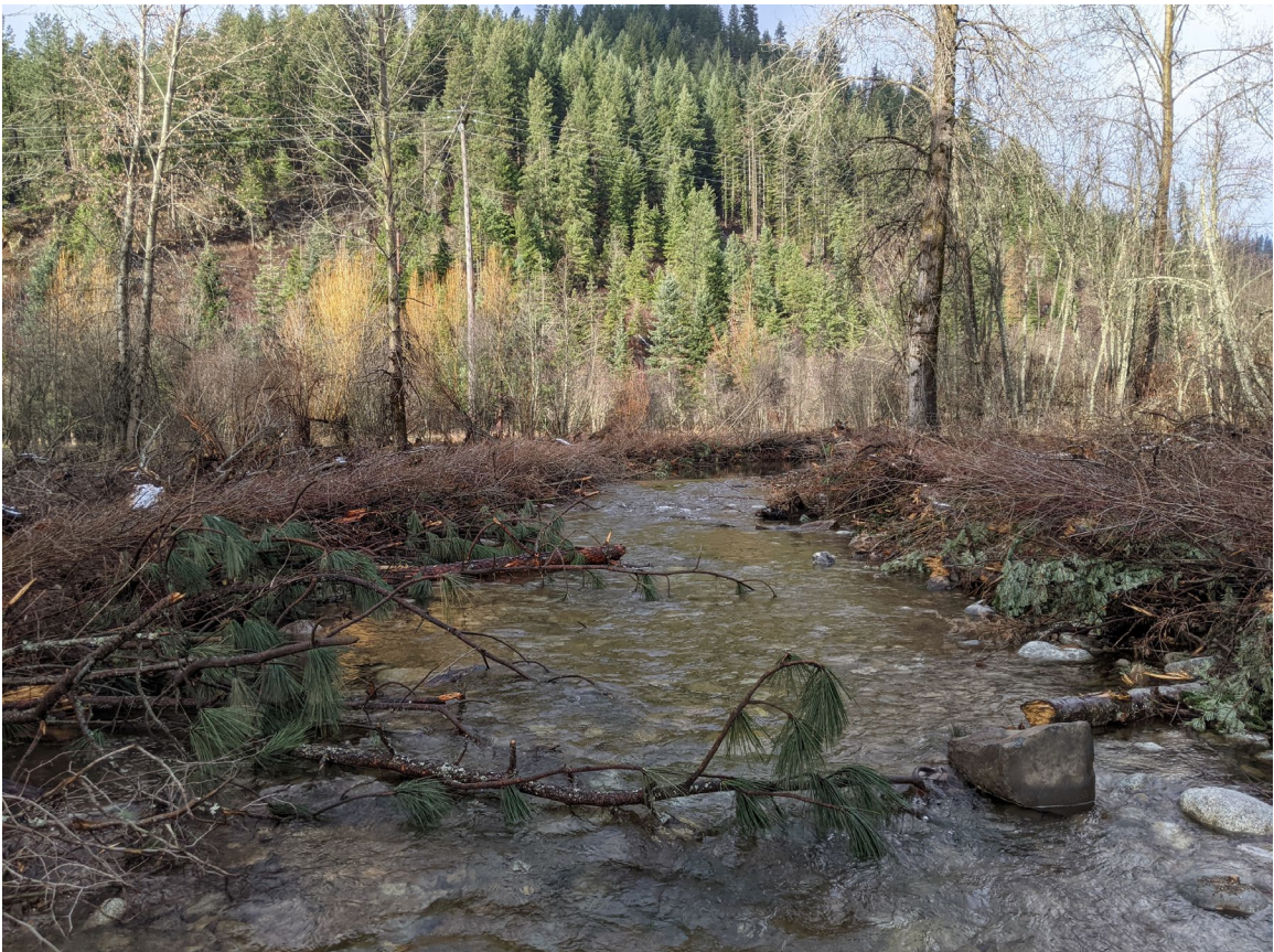
Photo 19: Post Construction. Installed Vegetated Wood Matrixes and constructed streambed upstream of property owner's structures. Facing upstream. ( PXL_20201125_172143597.jpg )
