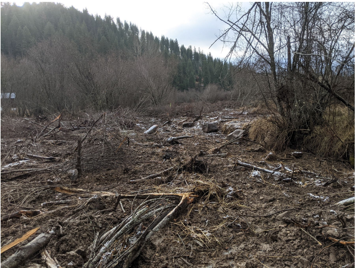
Photo 20: Post Construction. Installed floodplain treatment. Right bank, upstream of property owner's structures, facing downstream. ( PXL_20201125_172422048.jpg )
