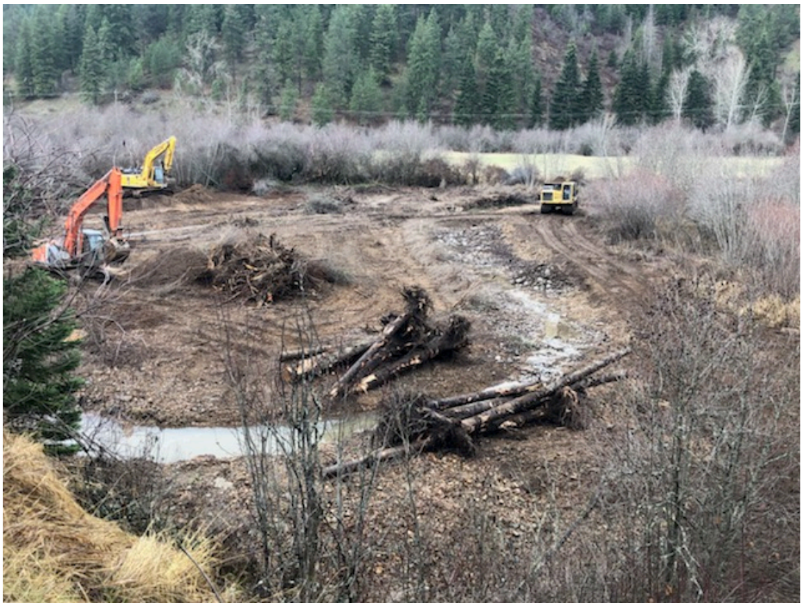
Photo 17: Construction. Recontouring of stream channel and floodplain enhancement, down stream of landowner property. Viewed from S Wolf Lodge Creek Rd. ( Road view.jpg )
