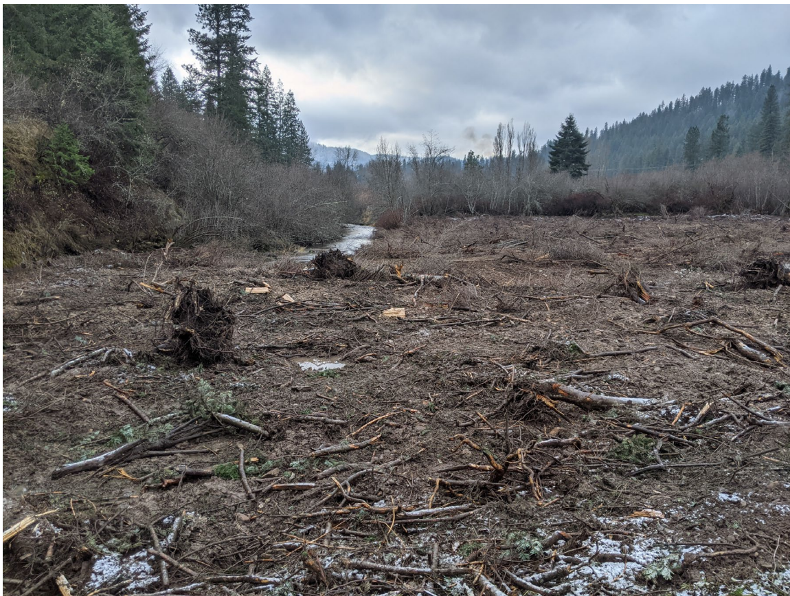
Photo 23: Post Construction. Floodplain treatment downstream of property owner's structures. Left bank, facing downstream. ( PXL_20201125_174233961.jpg )
