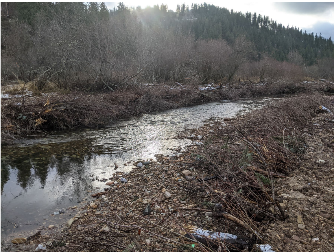
Photo 18: Post Construction. Installed Vegetated Wood Matrixes near upstream edge of project area, looking downstream. ( PXL_20201125_171322887.jpg )
